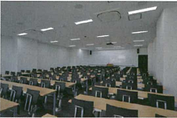
図2 講義室の照明 Fig.2 Lighting of lecture room.
